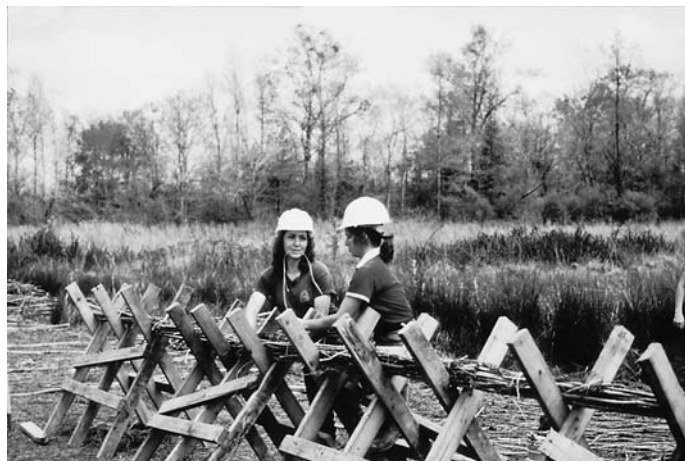
FIG. 1 Photograph of Live Fascine Fabrication (Tied Bundles, Not Installed and Resting on X-Shaped Sawhorses)
